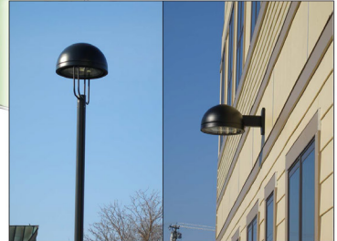
Exterior Lighting Metal halide lighting provides excellent efficiencies of 100 lumens/watt. The fixtures provide sharp cut off to reduce light pollution as well as photocell and time clock turn off capacities.
